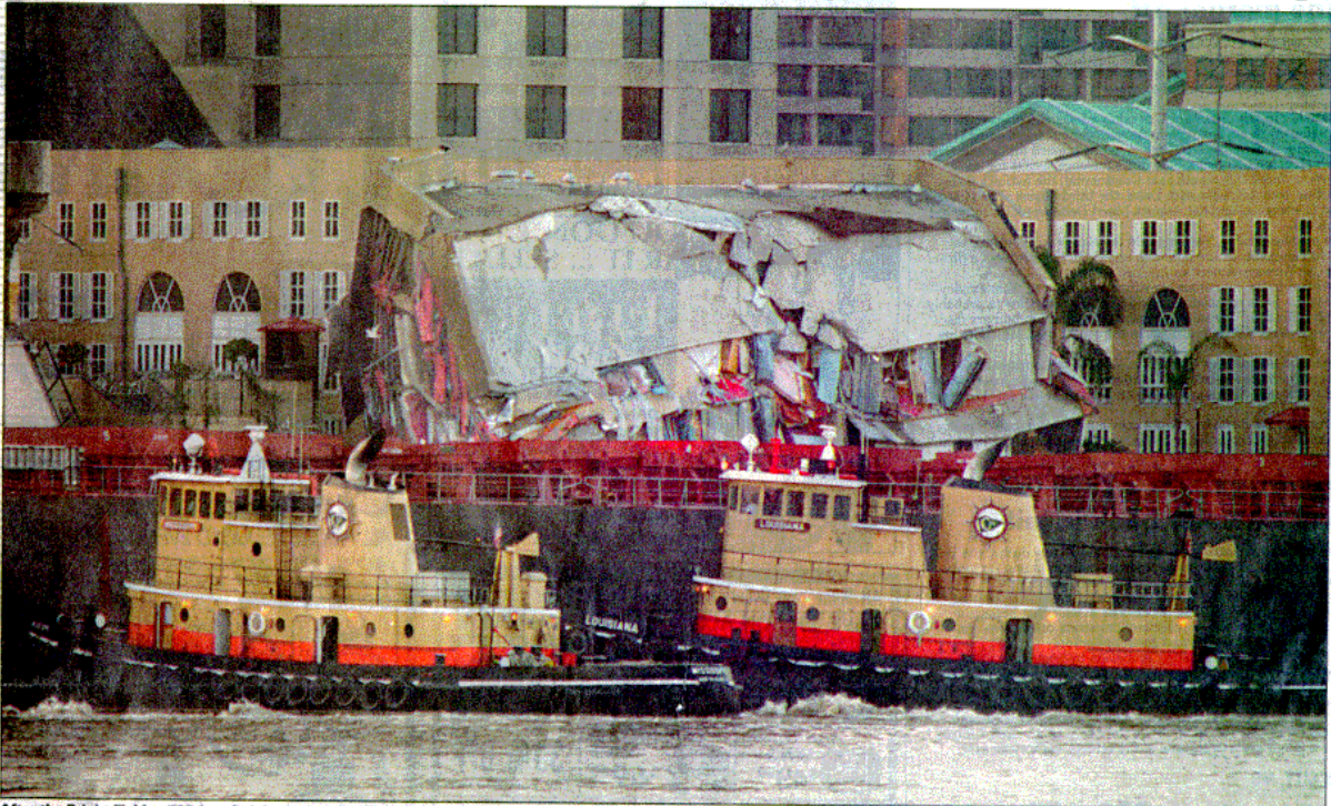
After the Bright Field, a 735-foot freighter, slammed into the Riverwalk mall Saturday afternoon, destroying shops and causing injuries and panic among holiday shoppers, tugboats secured the vessel against the devastated structure in hopes of preventing further collapse. The upper Poydras Street wharf, sections of the Hilton Hotel and some condos in One River Place also were damaged, officials said. STAFF PHOTO BY ELIOT KAMENITZ
